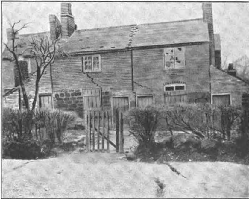
[This and the following illustrations are from photographs of the houses alluded to in 26 et seq. , and show them in successive stages of dilapidation.]
